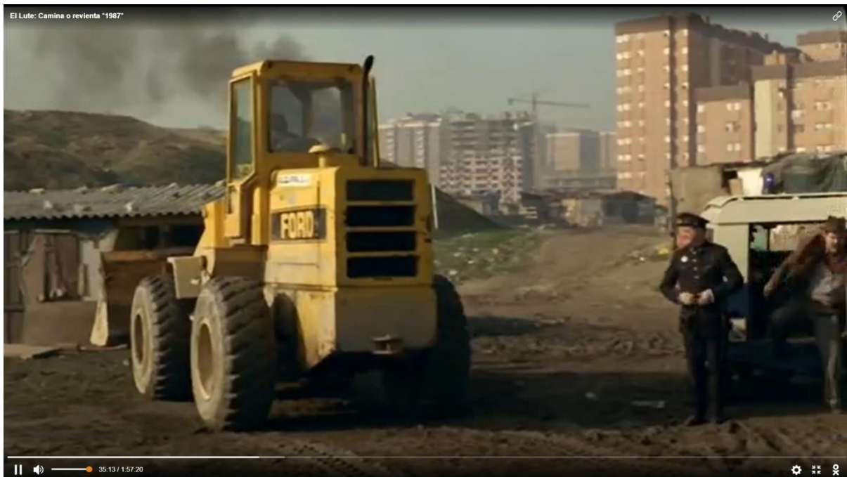
Fig. 28: El Lute I: Camina o revienta : the destruction of El Lute's self-constructed home with the modern high-rise blocks behind (minute 35).
