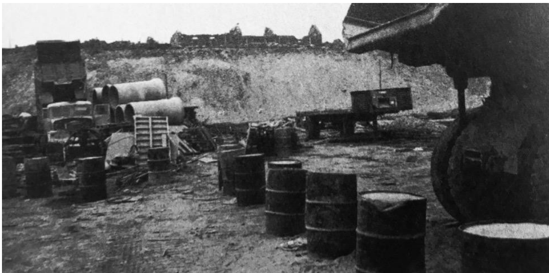
Fig. 22 'Shell construction site at Sullom Voe with crofts in the background' Caption for Untitled Fay Godwin, Photograph, 1975
